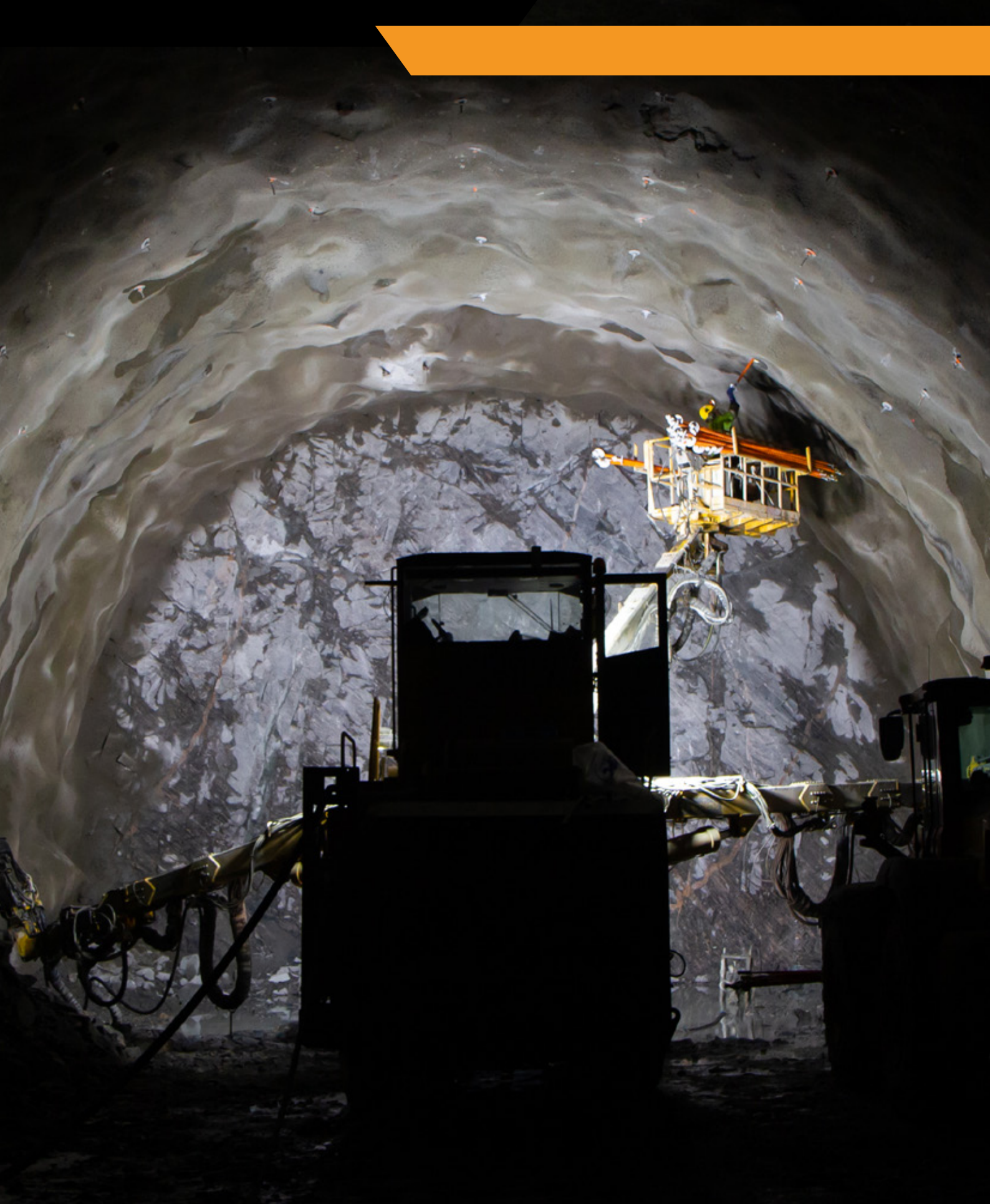
Rock support – M20 NC-Bolt Contractor: MossIA (Joint Venture Implenía Norge AS and Acciona Construction) Project: Railway tunnel, double track Sandbukta – Moss - Såstad, Norway
